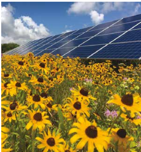
Forest City Solar Farm in Iowa produces approximately 6,000 MWh/year and is surrounded by pollinator friendly vegetation.
